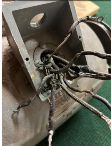
Failing HVAC equipment - motor driving our HVAC unit in the HS gym. The insulation is so old and brittle, it was falling apart from the wire.
