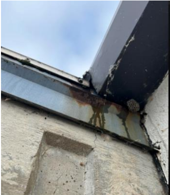
Aged and leaking gutters on the HS building caused water to run directly into the school creating damage to the Tech Ed ceiling.
